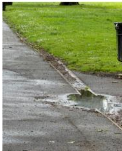
Figure 13. Pavement Condition in the Whitworth Park
